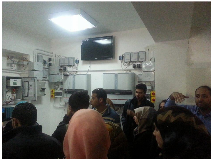
Fig. (2): Control and Monitoring Room of 30 kW Project.
