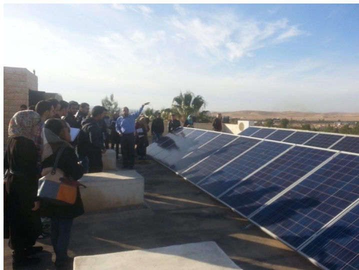
Fig.(3): Fixed PV Systems of 30 kW Project.
